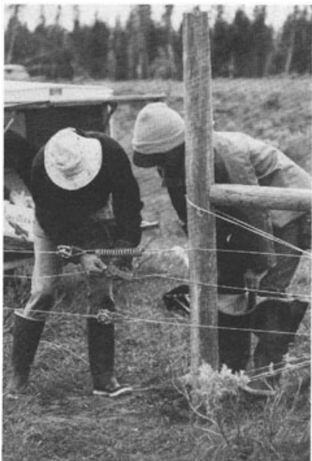
The final touches are added to the three strand wire high tension fence.
