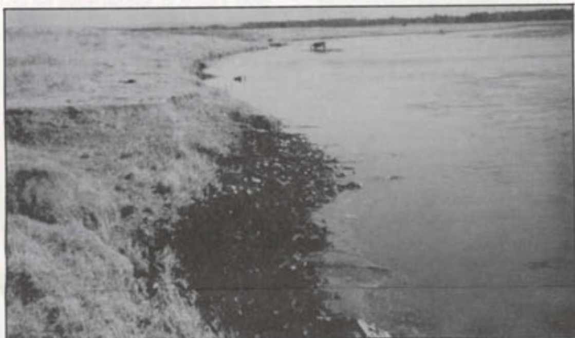
Bank damage at Harriman State Park - Fall 1987.
