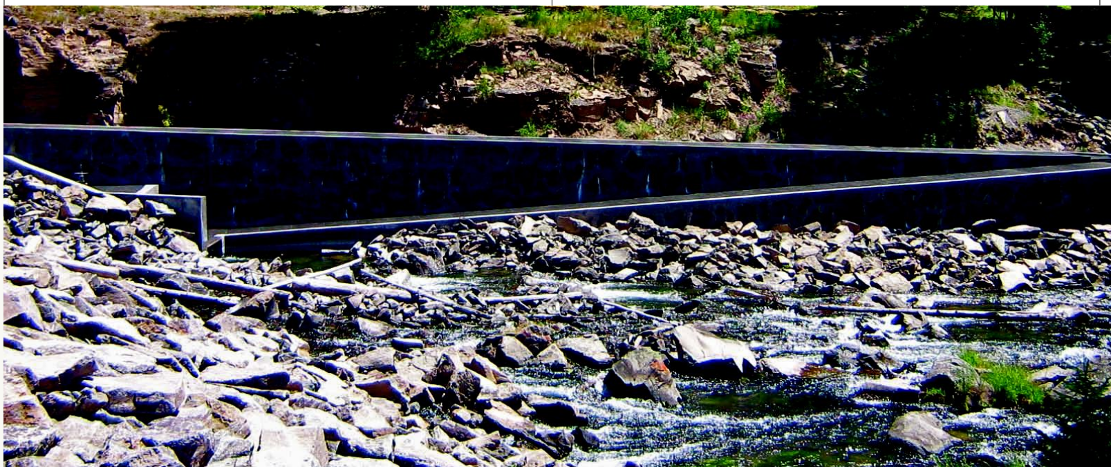
The new Buffalo River fish ladder was constructed in 2005. The objective of the ladder is to provide upstream fish passage and a connection to overwintering habitat. Photo: HFF
